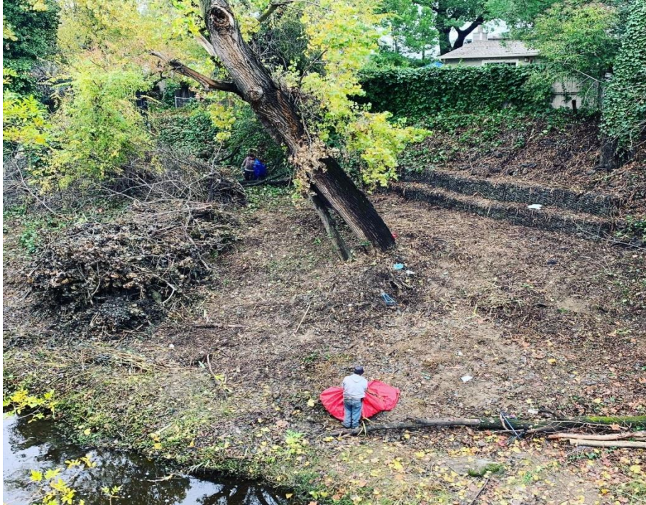
View 5. Walnut Creek site after clearance. The leaning cottonwood tree in the center provides a reference point to compare the cleared site with the pre-cleared site shown in View 4.
